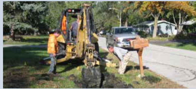
During the summer of 2016 seven major drainage projects were completed by the Joliet Township Road District.
